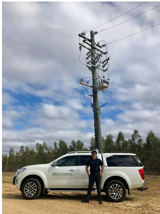
Rusty On Site at a NOJA Power OSM Recloser Installation
