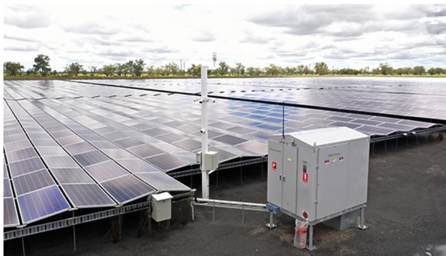
A NOJA Power GMK in Australia, connecting Solar generation to the distribution grid. © NOJA Power 2021
