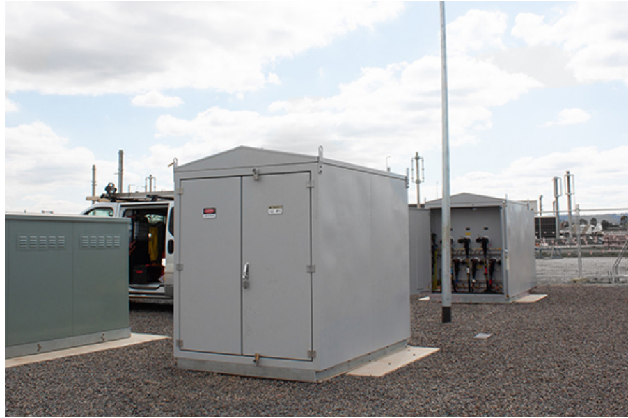
Two NOJA Power GMKs in Victoria Australia, connected in an Auto Changeover scheme supplying electricity to a railway substation © NOJA Power 2021
