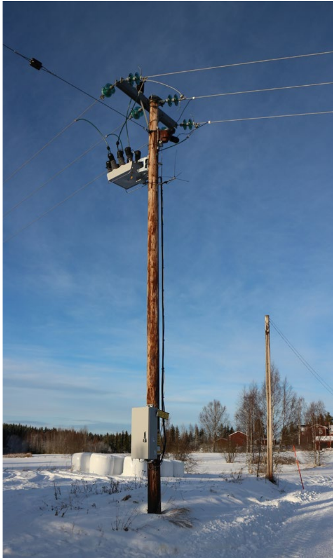
Typical installation design, OSM Recloser with RC Series Control
