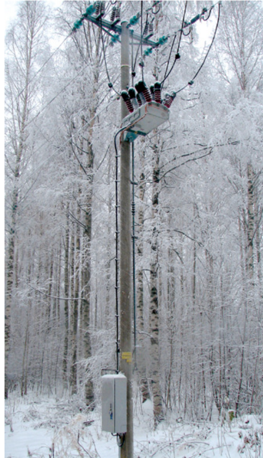
OSM recloser and RC10 Control and Communications Cubicle
