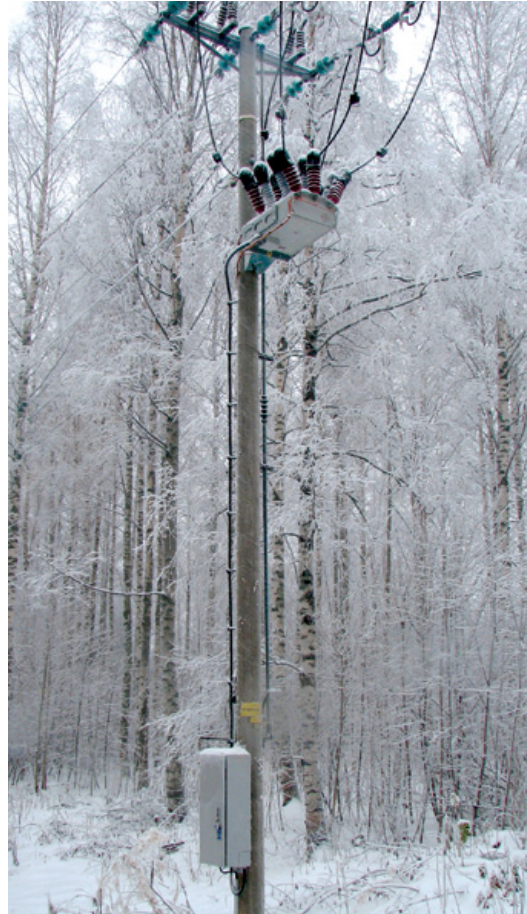
OSM recloser and RC Control and Communications Cubicle
