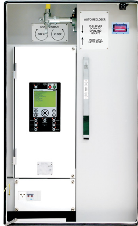
Control and Communications Cubicle
