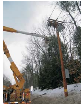
NOJA Power OSM Recloser pole-mount 200 series installation for PMLD
