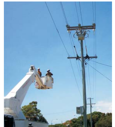
NOJA Power OSM Recloser installed as part of the ENERGEX five-year network upgrade program
